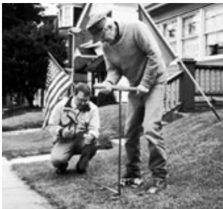
In the mid 1990's, Main Street Gettysburg began an interpretive wayside program. Jerry Bennett (standing) and Dr. Walter Powell are shown here, installing a wayside.
